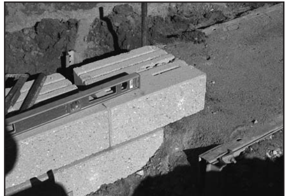
8. Step-up leveling pad and base course in six-inch increments when grade changes.
